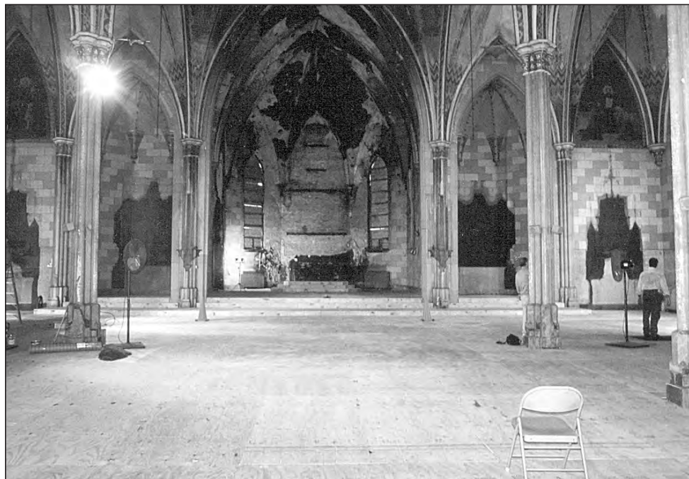
The inside of Sacred Heart of Jesus Church in Indianapolis is empty after an electrical fire on April 27 that started under the high altar. Protective flooring was laid for contractors to begin work on the walls and ceilings. Parishioners toured the church after Masses on Labor Day weekend.
