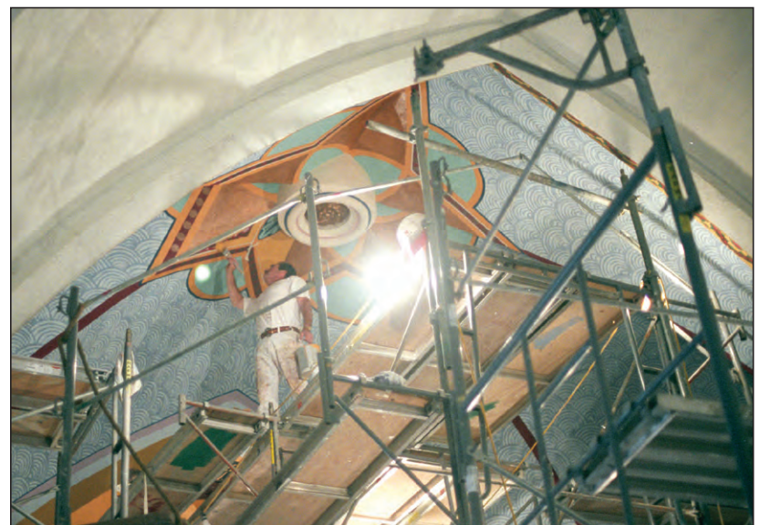
This scaffolding reaching to the church ceiling was recently removed from the interior of Sacred Heart of Jesus Church.
