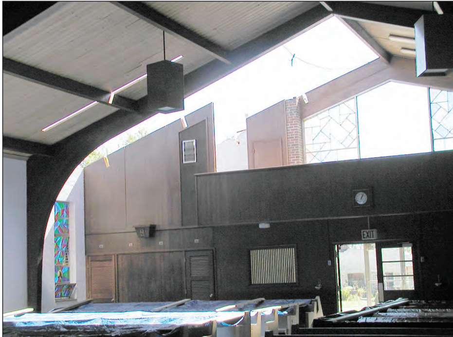
St. Martin of Tours Church in Martinsville sustained major damage after a tornado tore the roof off on Sept. 20. The roof of nearby Sexton Hall was also damaged. No one was injured at the church.
