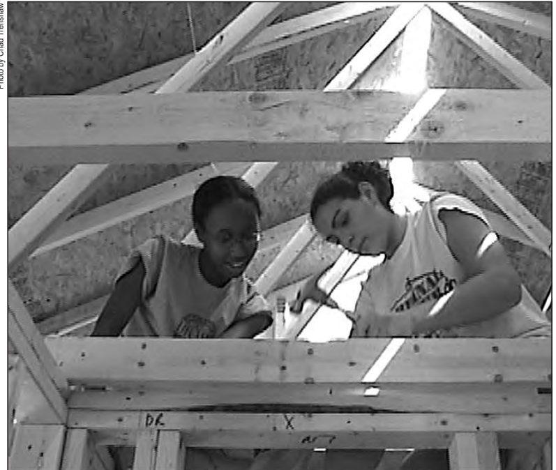
Cardinal Ritter High School juniors Kellye Sibley and Lauren Hernandez of Indianapolis work to build a home for Habitat for Humanity. Students from Cardinal Ritter, Father Thomas Scecina Memorial and Bishop Chatard high schools in Indianapolis worked together to build the home for a needy family.
