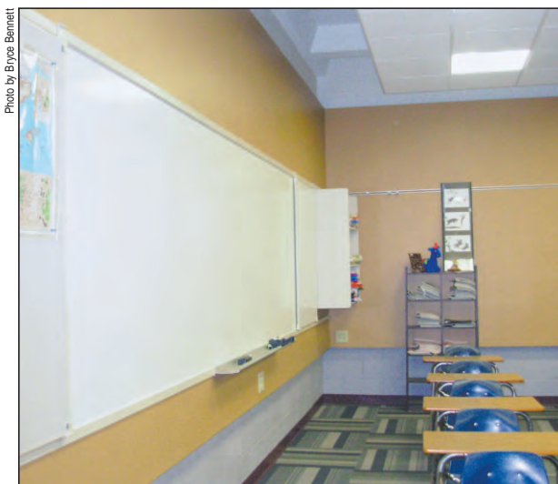
Remodeled classrooms are part of an ongoing renovation program at Father Thomas Scecina Memorial High School in Indianapolis.
