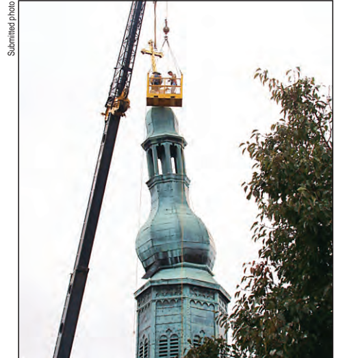
Workers use a crane to assess the damage to the steeple at St. Mary Church in New Albany on Sept. 15.
