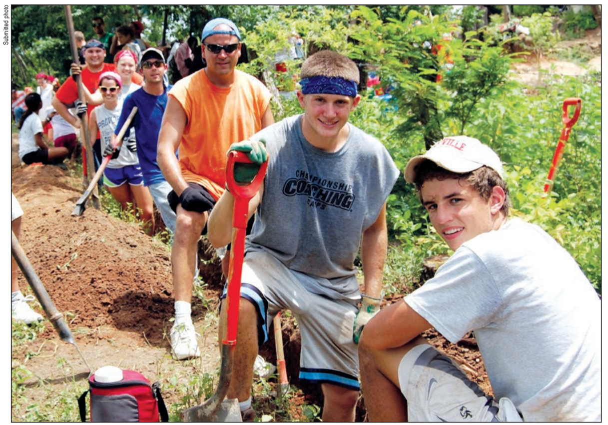
Volunteers from Our Lady of Providence Jr./Sr. High School in Clarksville take a break from digging a trench to bring clean running water to outlying villages in Nicaragua in the summer of 2012. From left, senior Lloyd Lashley, junior Abby Spitznagel, junior Megan Gilland, 2012 graduate Elliott Happel, Spanish teacher Alan Mathews, junior Trey Embry and junior Austin Happel.
